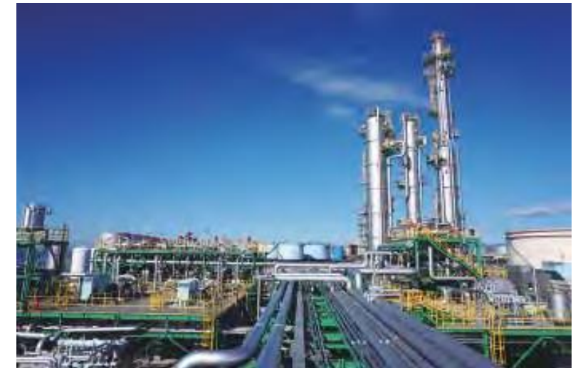
CCS Demonstration Project in Tomakomai < Source > “The CCS Demonstration Project is underway in Tomakomai” (Japan CCS Co., Ltd.)
